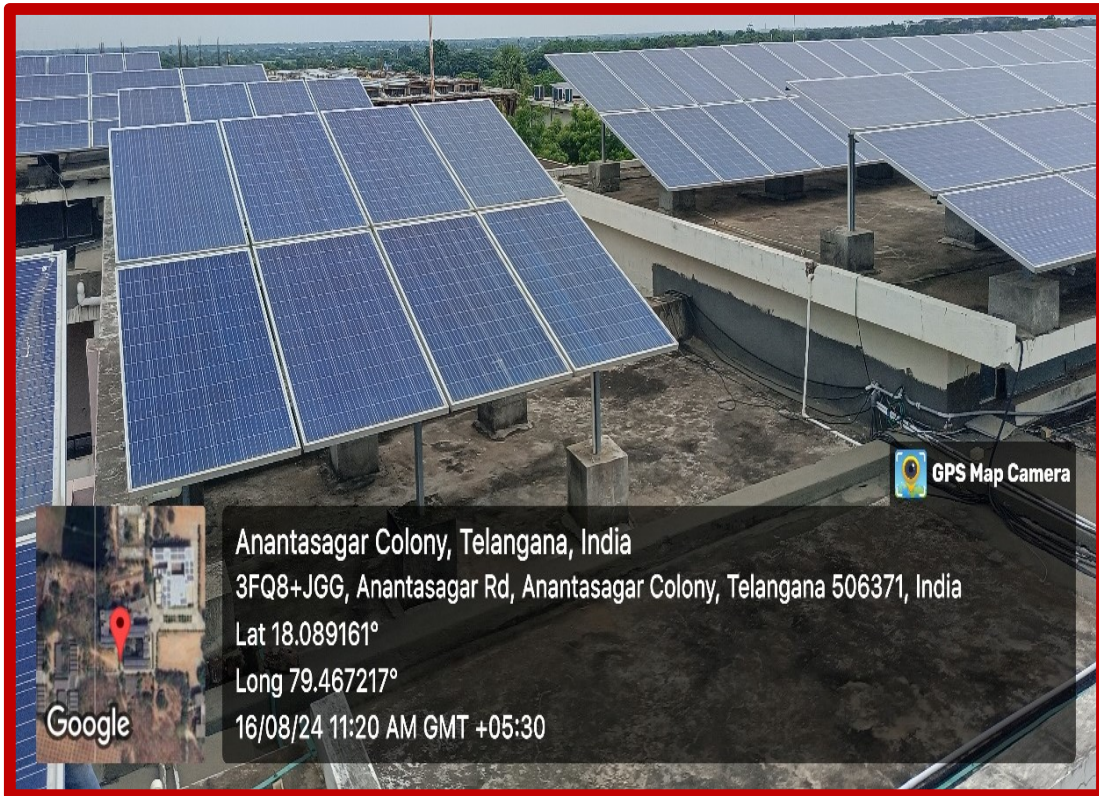
Grid-Connected Rooftop Solar Photovoltaic (SPV) Systems at Block 1
