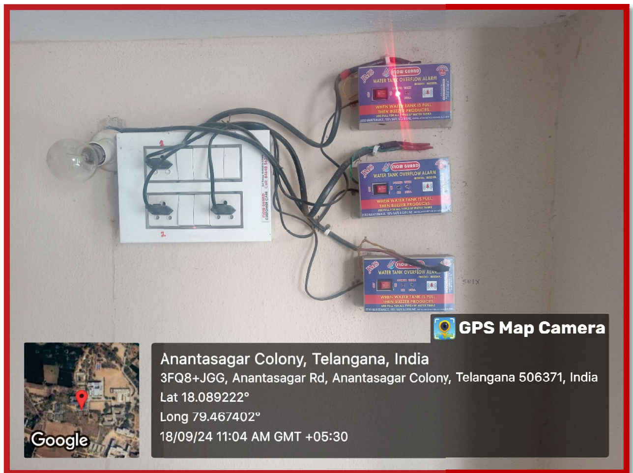
Sensor based Water tank Overflow Alarm
