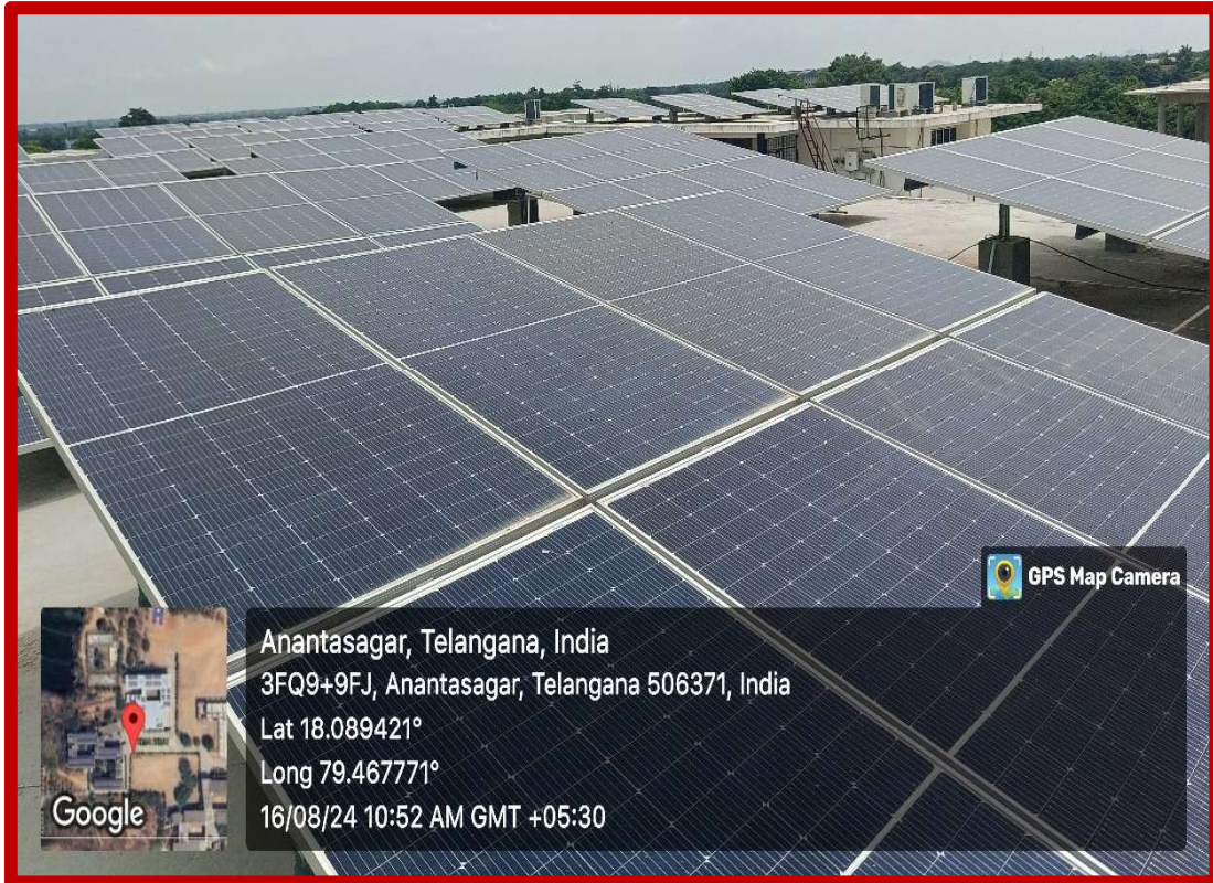
Grid-Connected Rooftop Solar Photovoltaic (SPV) Systems at SRIX
