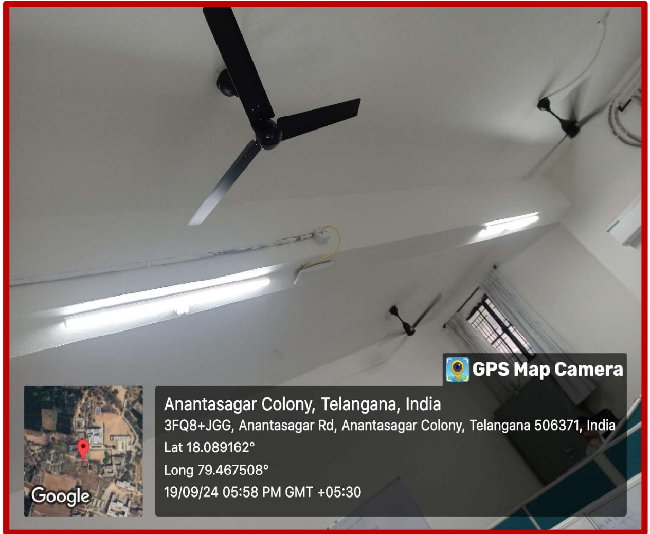
LED Bulbs and Energy Saving BLDC fans in Staff Room
