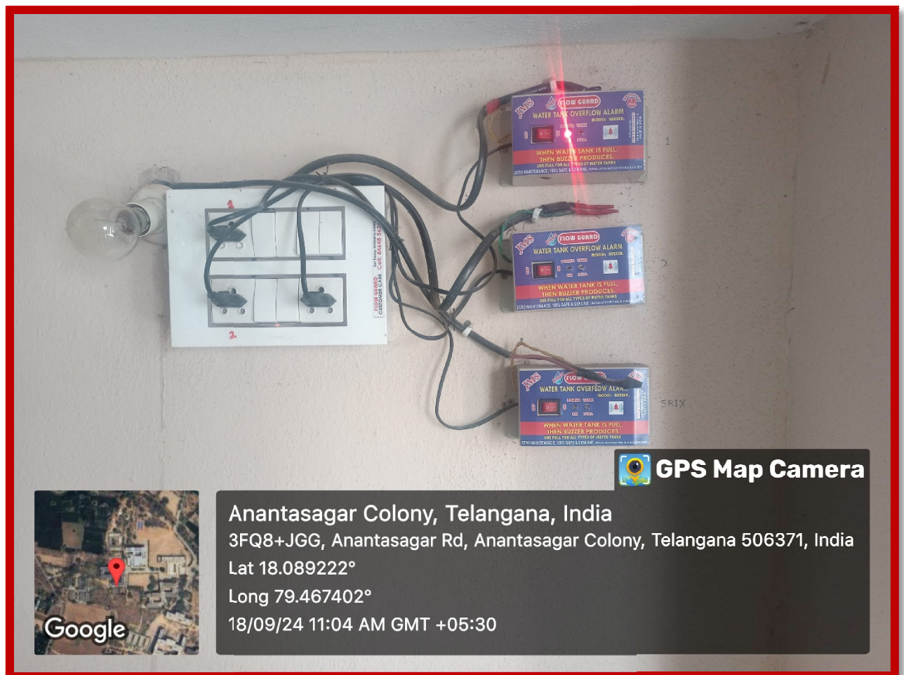
Sensor based Water tank Overflow Alarm
