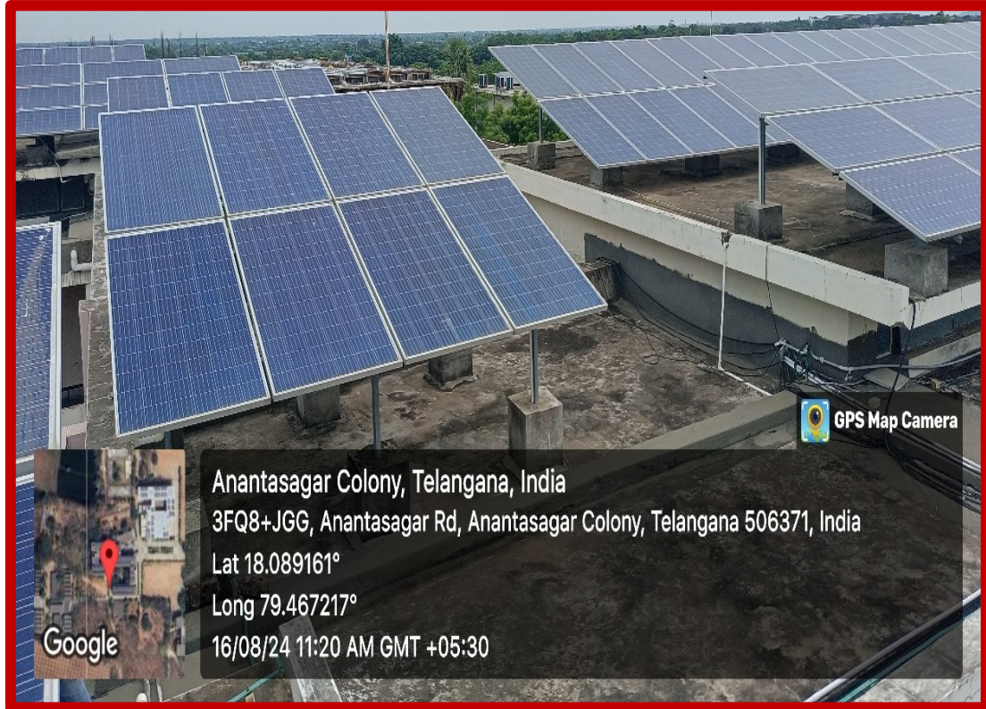
Grid-Connected Rooftop Solar Photovoltaic (SPV) Systems at Block 1
