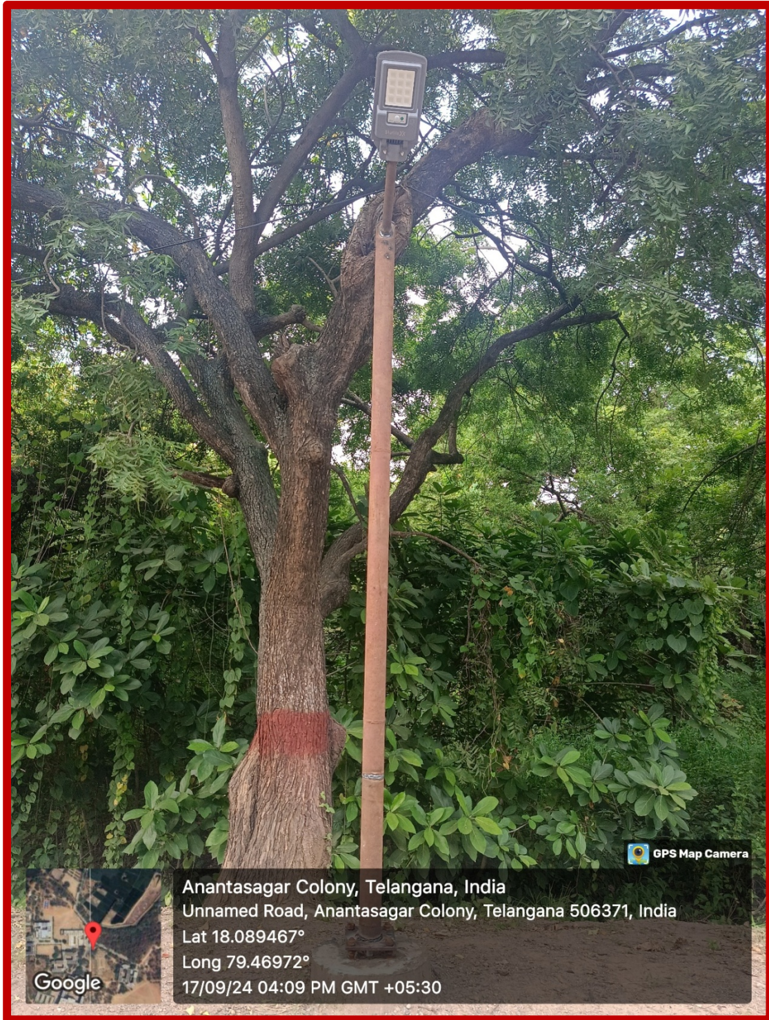
Sensor Based Solar Street Light
