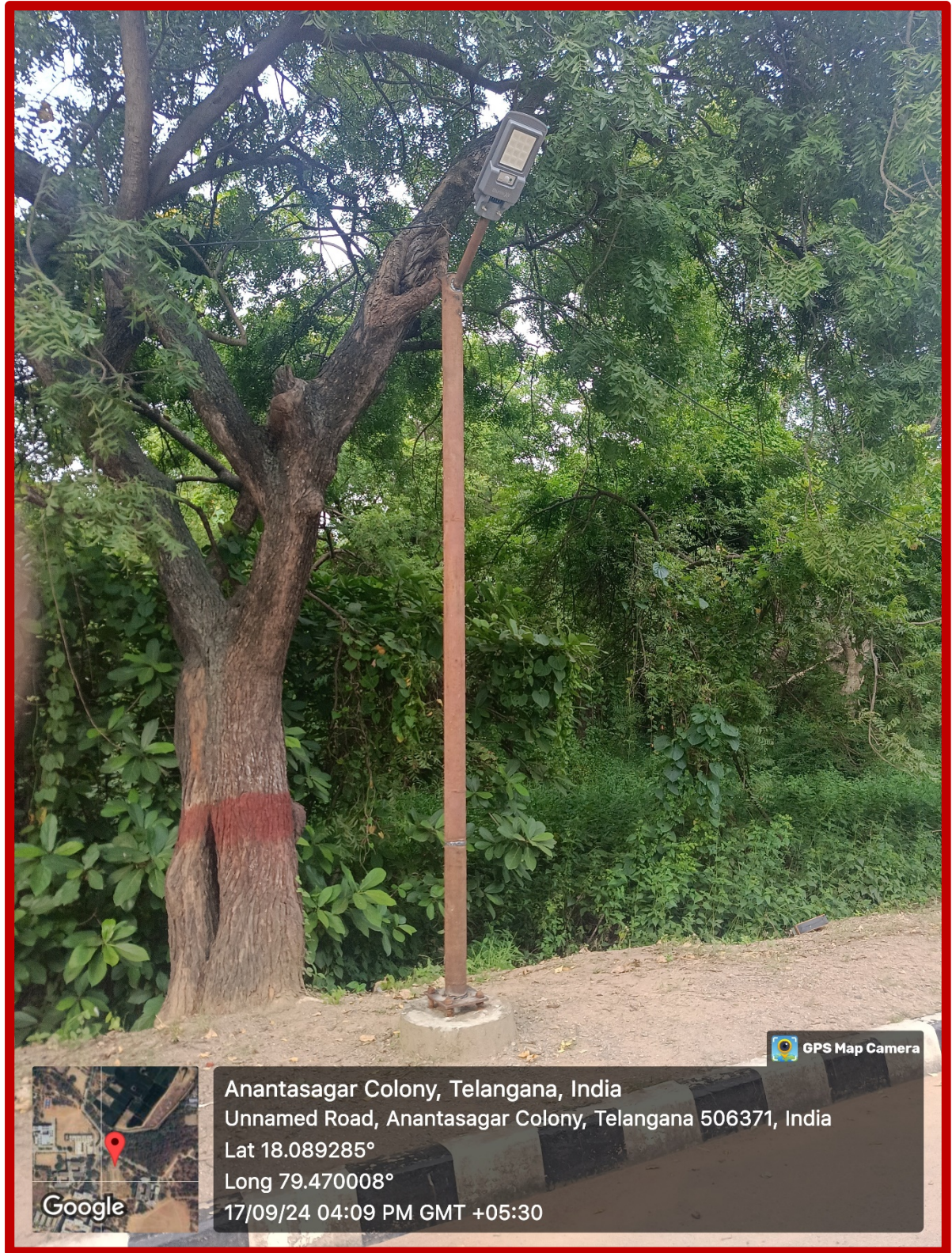
Sensor Based Solar Street Light
