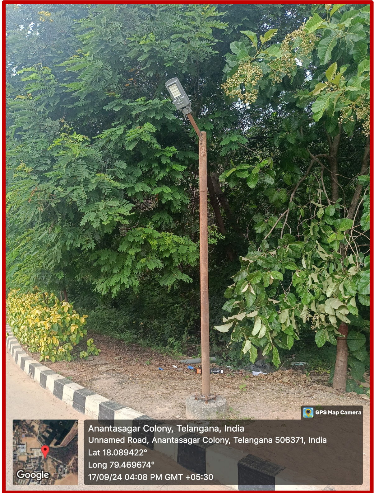
Sensor Based Solar Street Light
