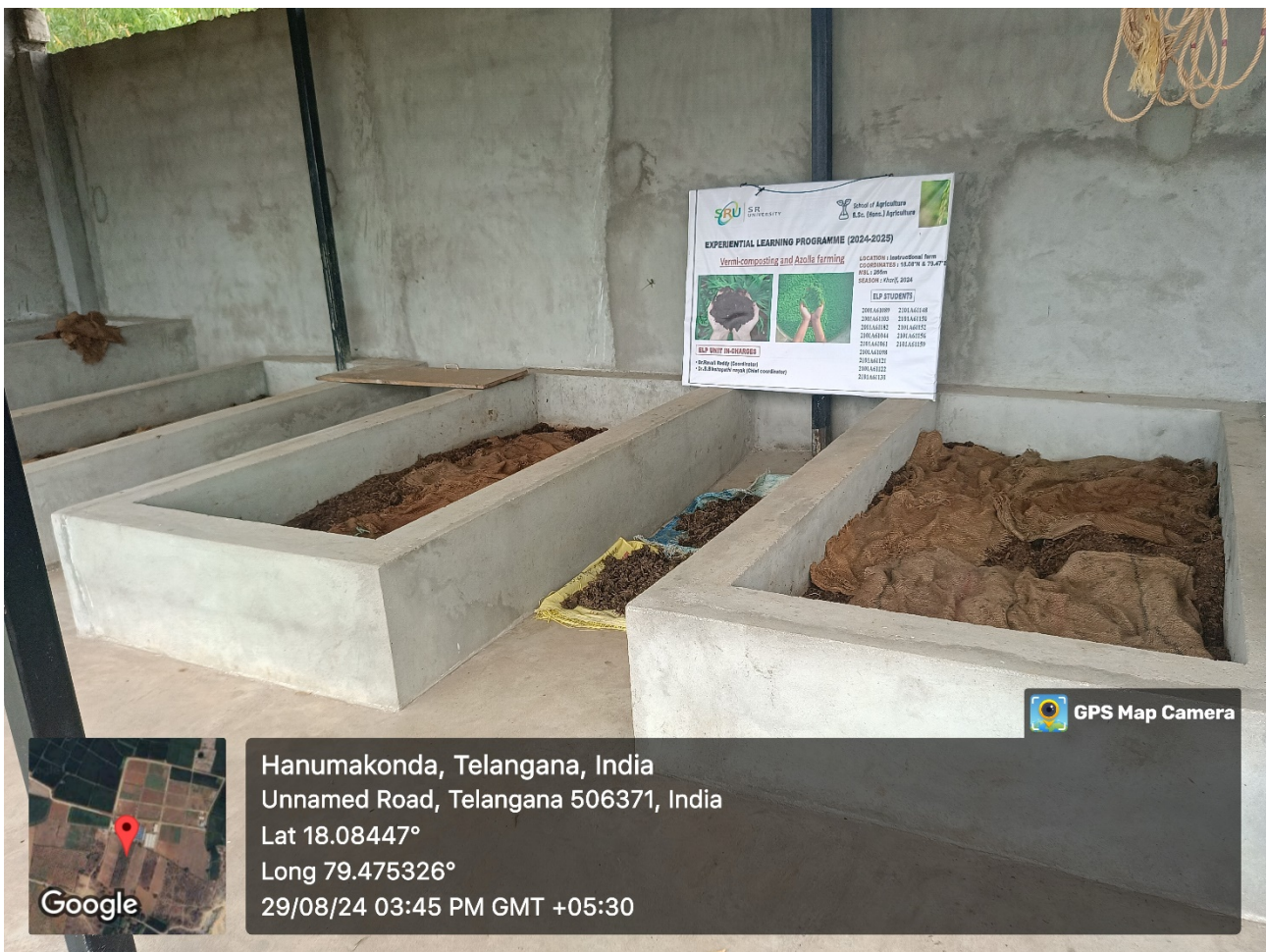
Compost Pits for maintaining the Sludge
