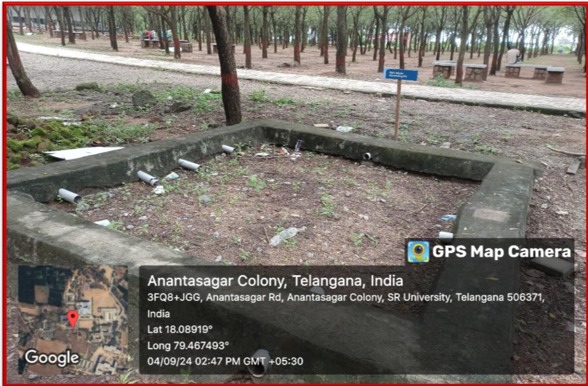
Rain Water Harvesting Pit: Block II South West Corner
