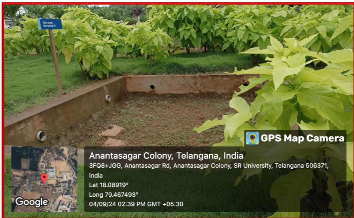
Rain Water Harvesting Pit: Block 1 North East Corner
