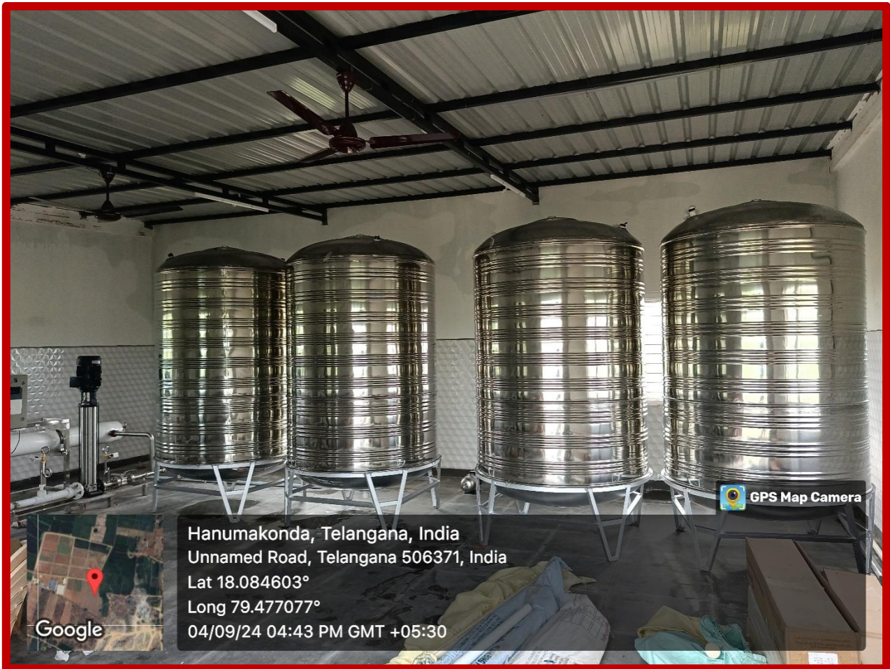
Water Tanks for Filtered Water
