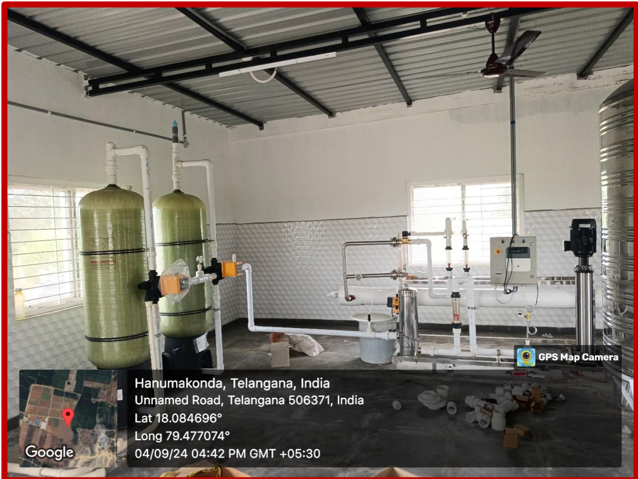
RO Water Treatment System
