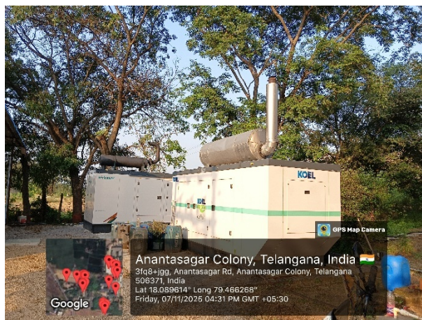
Biodiesel Generator Unit
